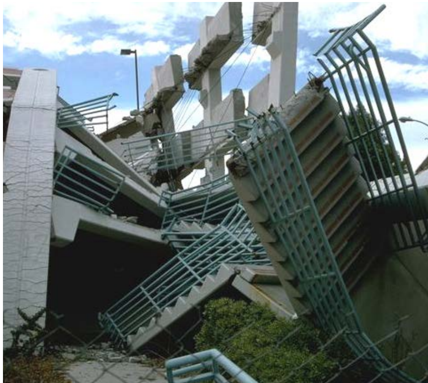
An earthquake destroyed this building.
