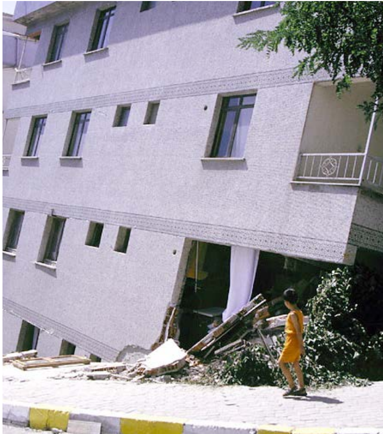
Earthquakes can damage or even destroy buildings.
